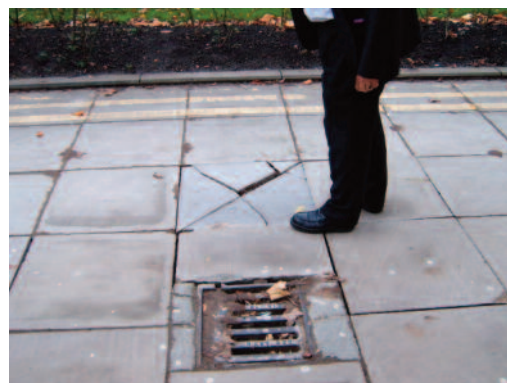
If you see it, please report it! Let the Estates Helpdesk know about broken or loose paving
