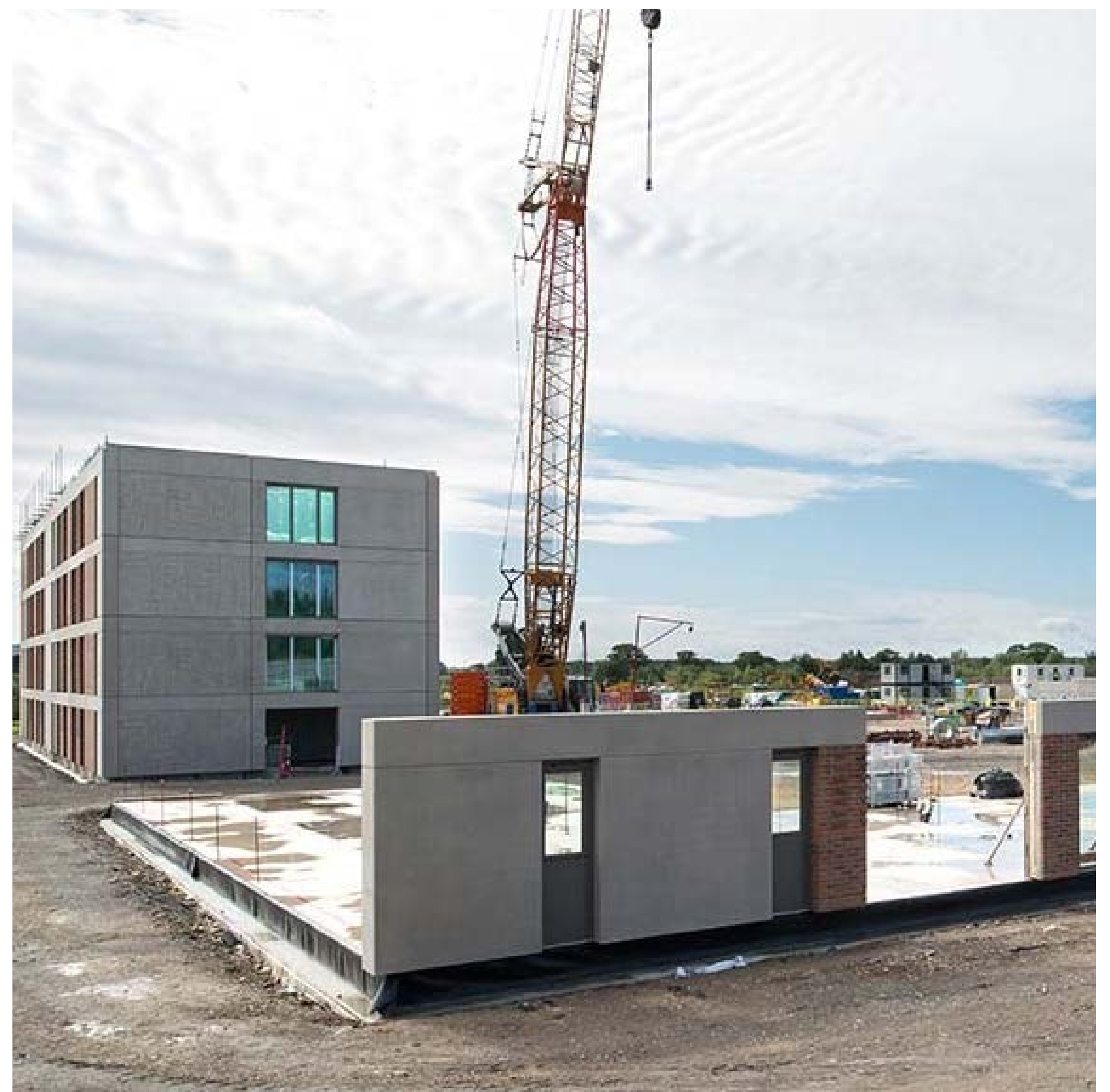
An example of panels, which were constructed within a factory environment, being installed as part of a methodical construction programme. This process significantly reduces deliveries to site
