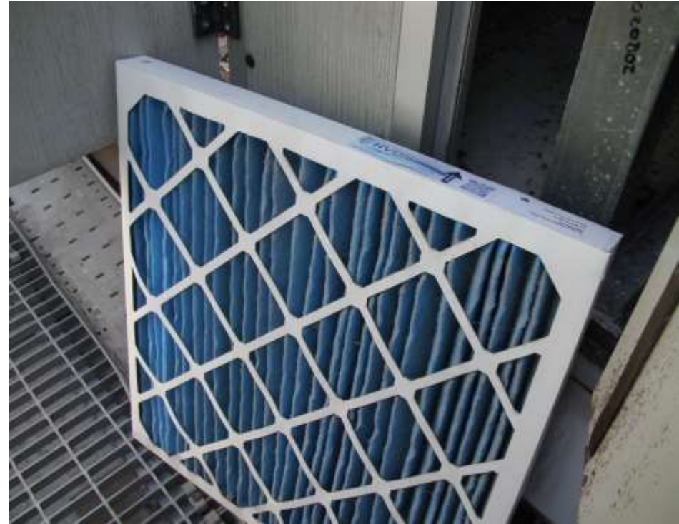
Filters for Air Handling Units – part of maintenance schedule but found to be absent in one site
