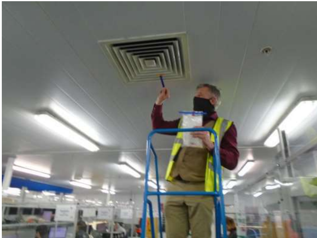
Air handling and ceiling ventilation
