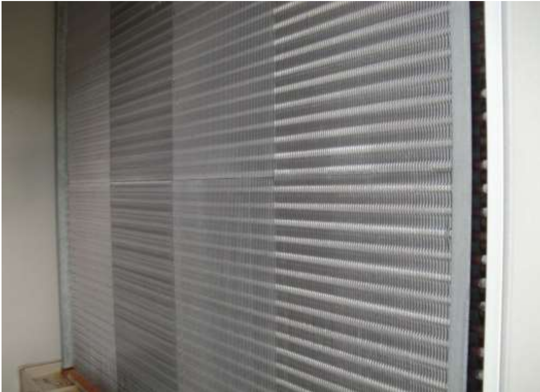
Air Handling Units – for chilling air and recirculation to high care production areas
