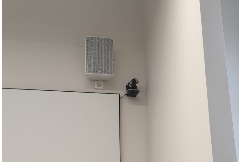
Wall mounted "room" camera
