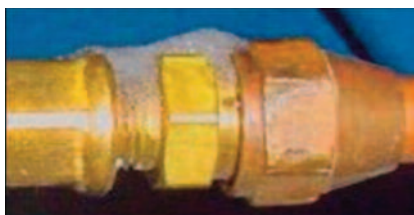
Bubbles form if a leak is present
