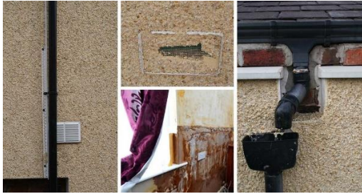
Figure 3. Photos illustrate the outcomes from the retrofit project in Preston that affected 390 homes. The occupiers reported water penetration, damp and mould. Some of them were forced to vacate the property. Source: Passive House Plus , 2018 26 .
